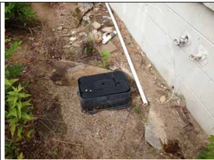
11. View of the water meter.
