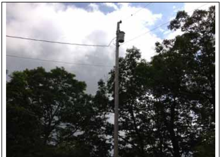
12. View of the onsite pole-mounted electrical transformer.
