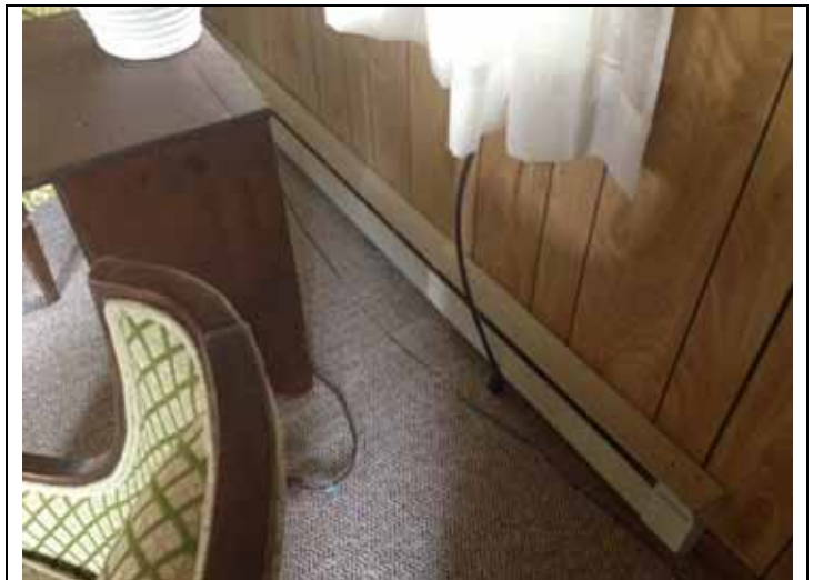
24. View of a heating unit in the home.
